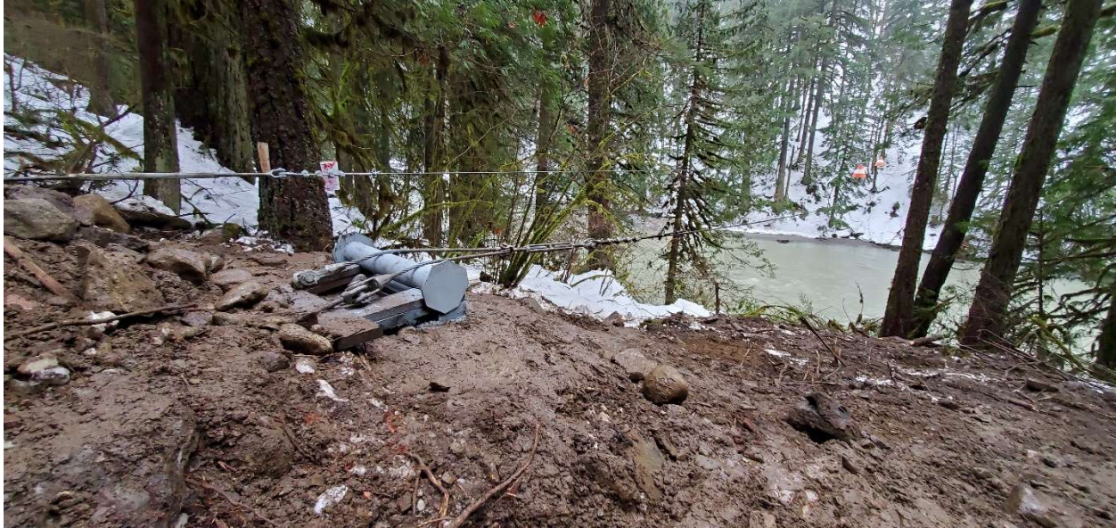
Figure 4: Example of Pipe Support
