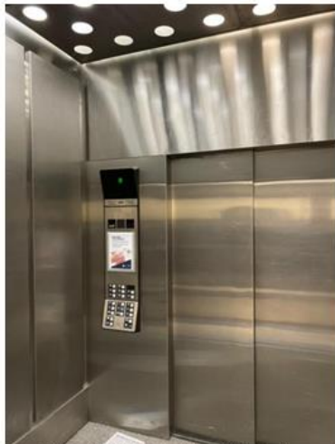
Picture 5: Picture inside freight elevator
