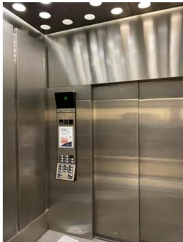
Picture 5: Picture inside freight elevator
