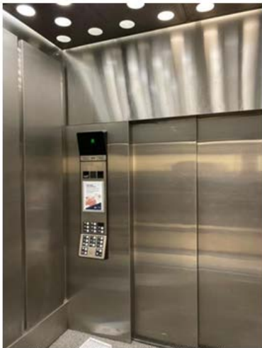
Picture 5: Picture inside freight elevator
