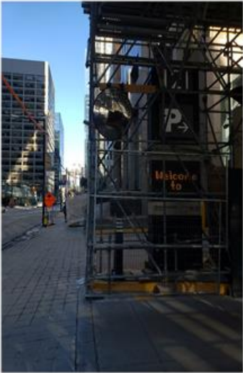
Picture 1: Picture from street of side of 121 King Street West where loading dock is located.
