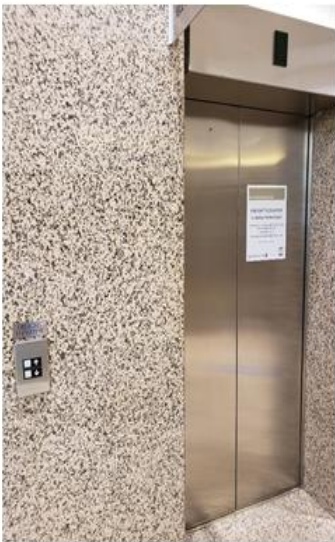
Picture 5: Picture freight elevator
