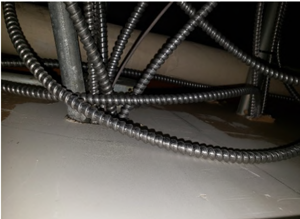
Photograph 13: Loc 5; Ceiling cavity; Area proposed to be impacted by renovation work; No asbestos detected in drywall joint compound
