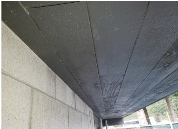
Photograph 20: Loc 6 - Exterior; Lead-containing black paint on wood soffit (590 ppm lead)
