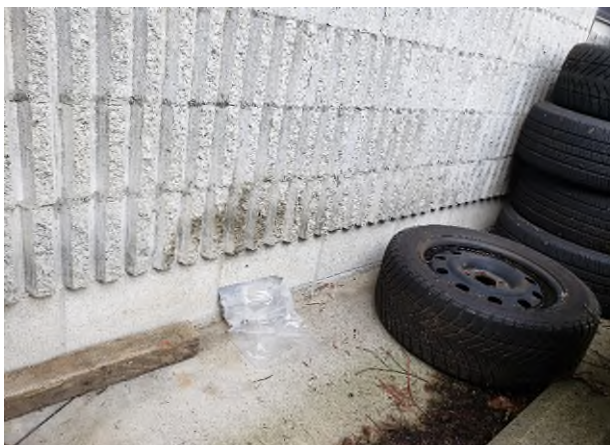
Photograph 5: Building exterior (east); no vermiculite observed in masonry wall after performing destructive test
