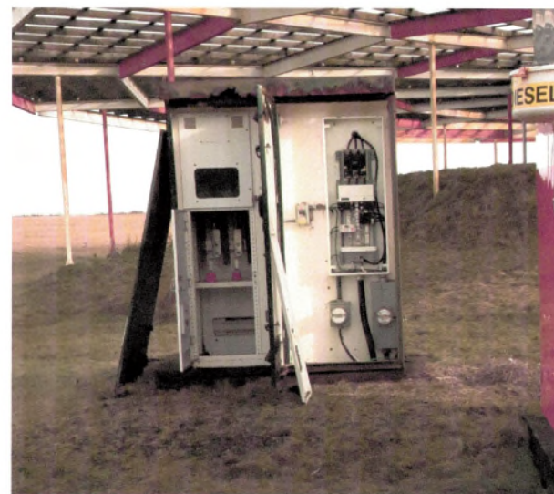
2 EXISTING SUBSTATION E07
