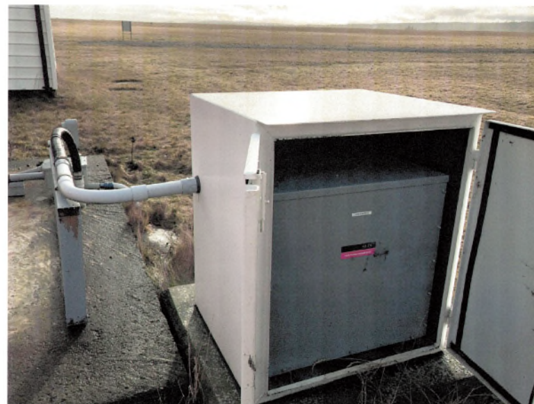
4 AWOS TRANSFORMER AND ABOVE GRADE FEEDER CONDUIT E07
