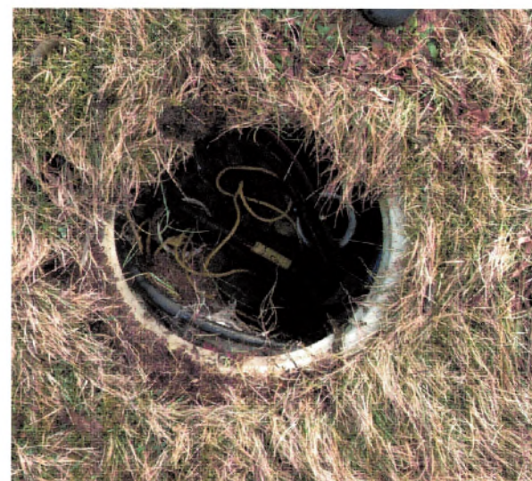
6 EXISTING SPLICE BOX 'PB-04' E07
