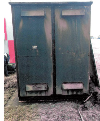
3 EXISTING SUBSTATION E07
