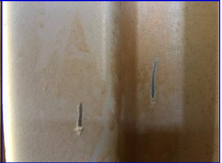
5.08 Fingernail removes paint to siding
