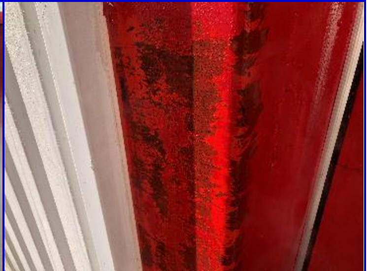
5.24 Tightly adhered paint
