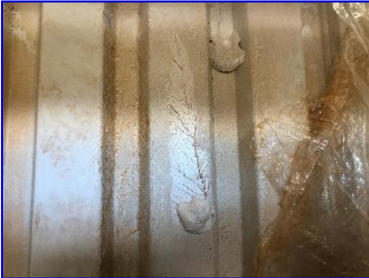
5.09 Paint delaminates to siding when plastic removed
