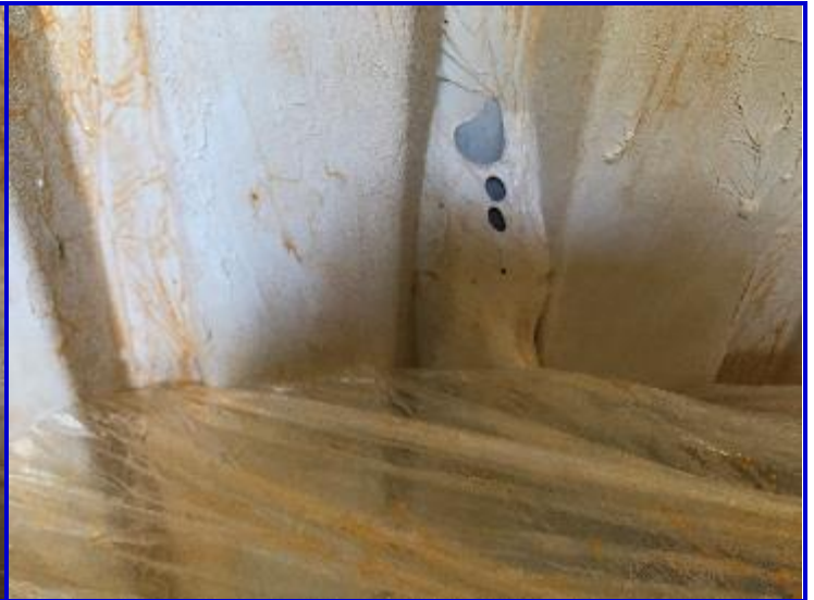
5.10 Paint delaminates to siding when plastic removed
