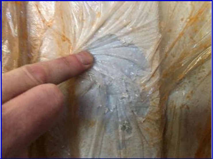
5.04 Paint debonded from the siding
