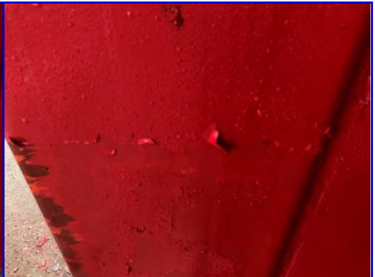
5.26 Loose top layer of paint
