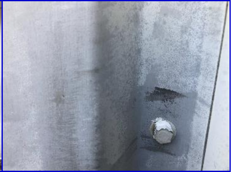
5.04 incomplete paint removal
