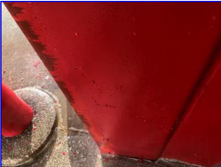
5.25 Loose top layer of paint
