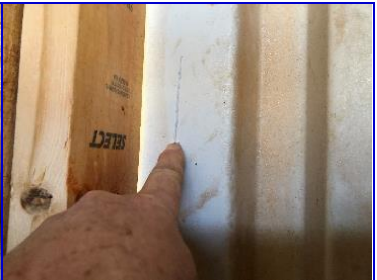
5.06 Fingernail removes paint to siding
