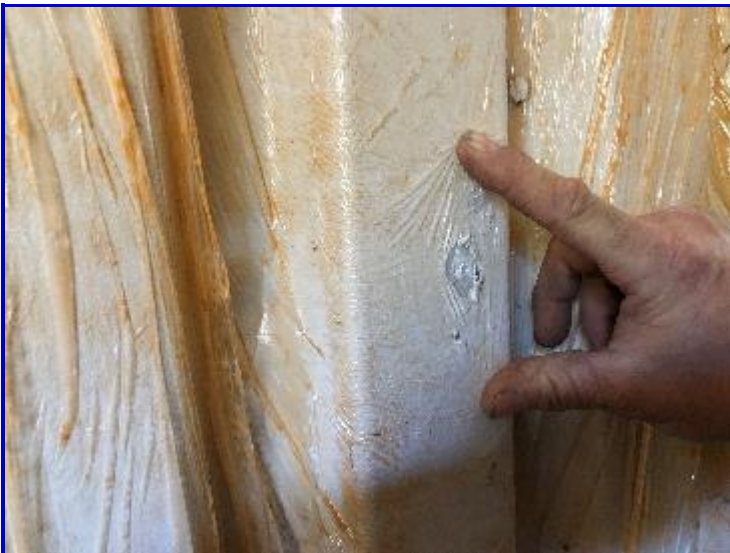
5.05 Paint debonded from the siding
