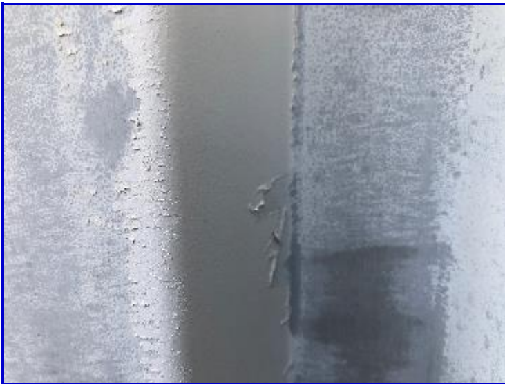
5.05 incomplete paint removal
