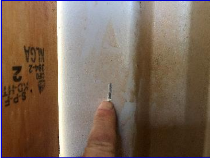
5.07 Fingernail removes paint to siding
