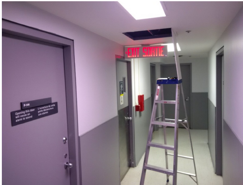
Photo 3: Typical drywall in the P1 level. All drywall joint compound is to be treated as asbestos-containing.
