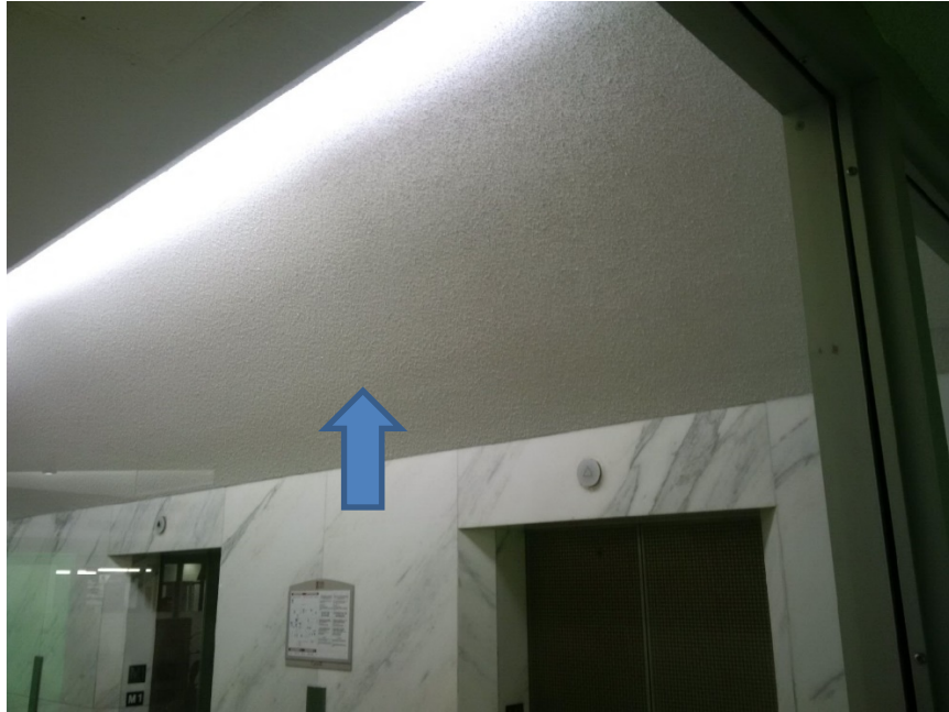
Photo 1: Ceiling stipple on drywall adjacent to elevators does not contain asbestos. Drywall joint compound under stipple does contain asbestos.
