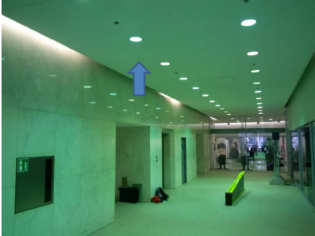
Photo 5: Ceiling stipple and drywall joint compound on elevated ceilings in west tower contain asbestos.
