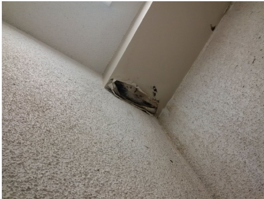
Photo 2: Drywall ceiling bulkhead with water damage and suspected mould growth in the west tower P1 level stairwell corridor. Drywall joint compound is suspected to contain asbestos. Textured plaster walls do not contain asbestos.
