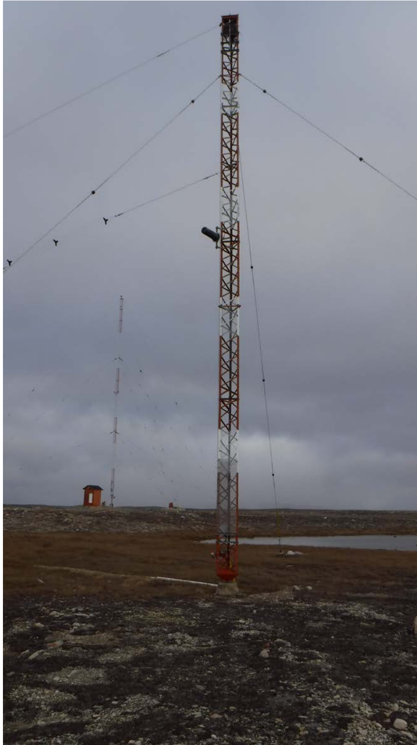
Figure 5: Existing M10 tower and VHF Antenna
