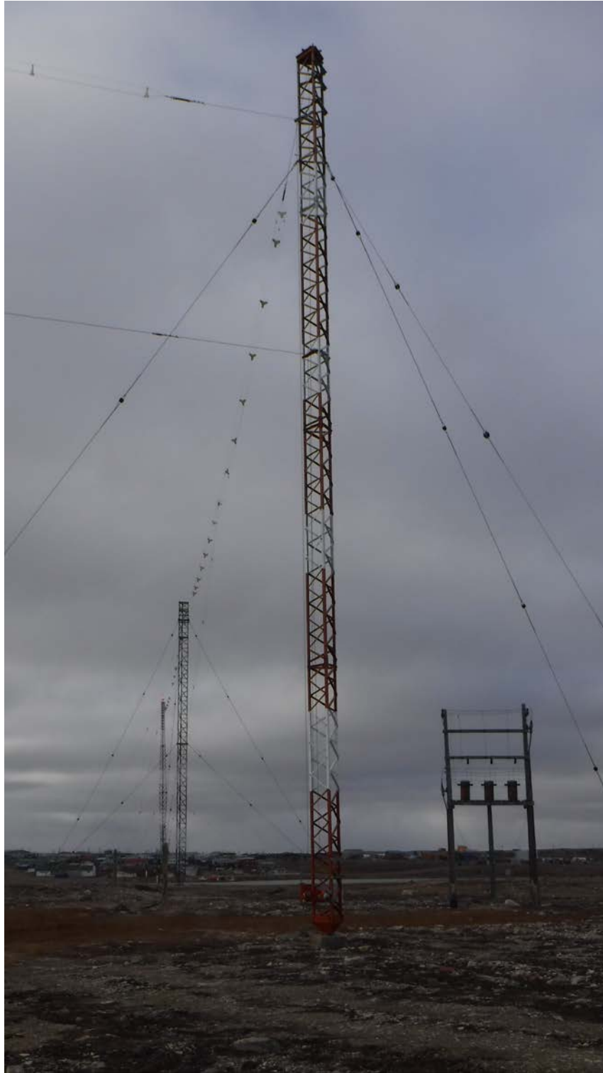
Figure 6: Existing M6, M5 and M4 towers
