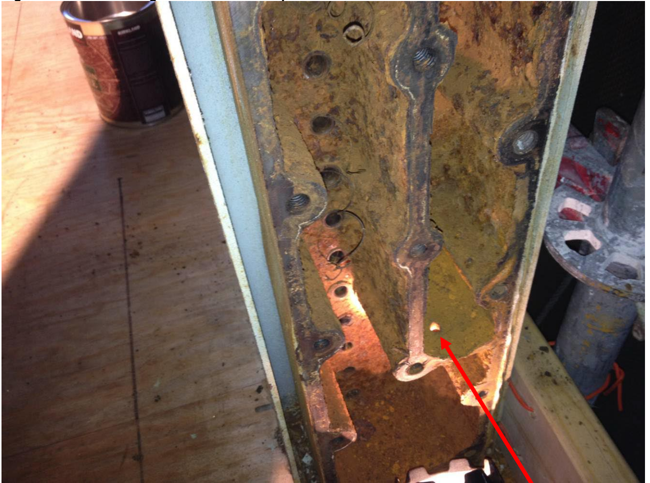
Figure 14: Heat Exchanger Coil Internal Weep Hole
