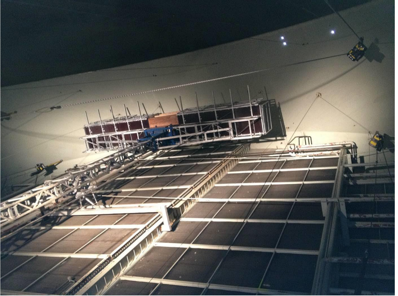
Figure 12: Upstream Mast Climber Near the Top. (Shown partially assembled, not full width)
