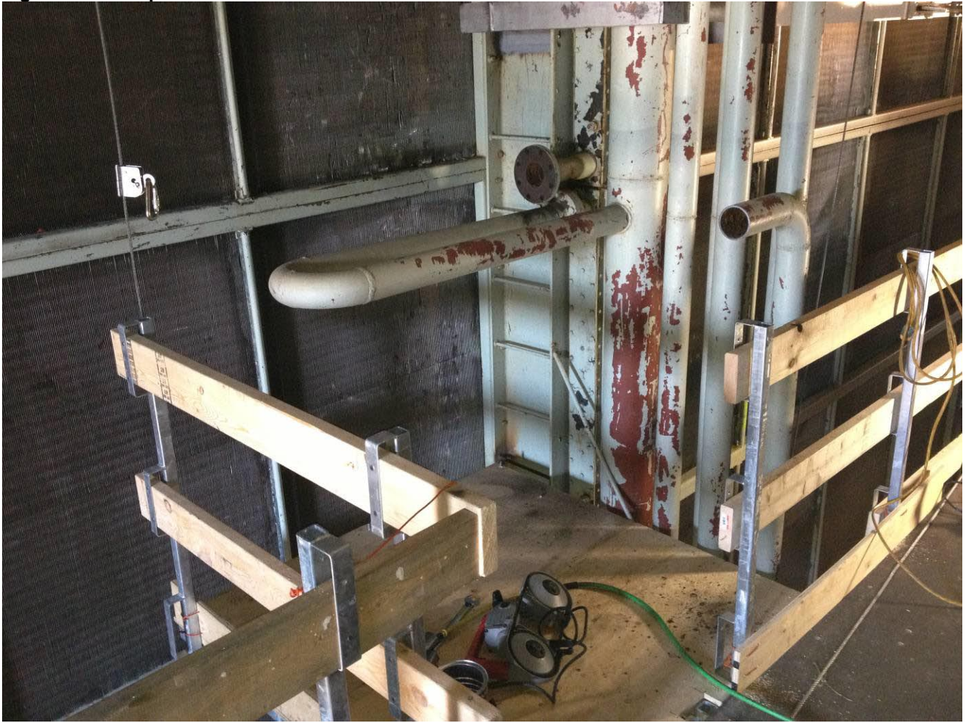
Figure 13: Example of a MCWP Platform Extension
