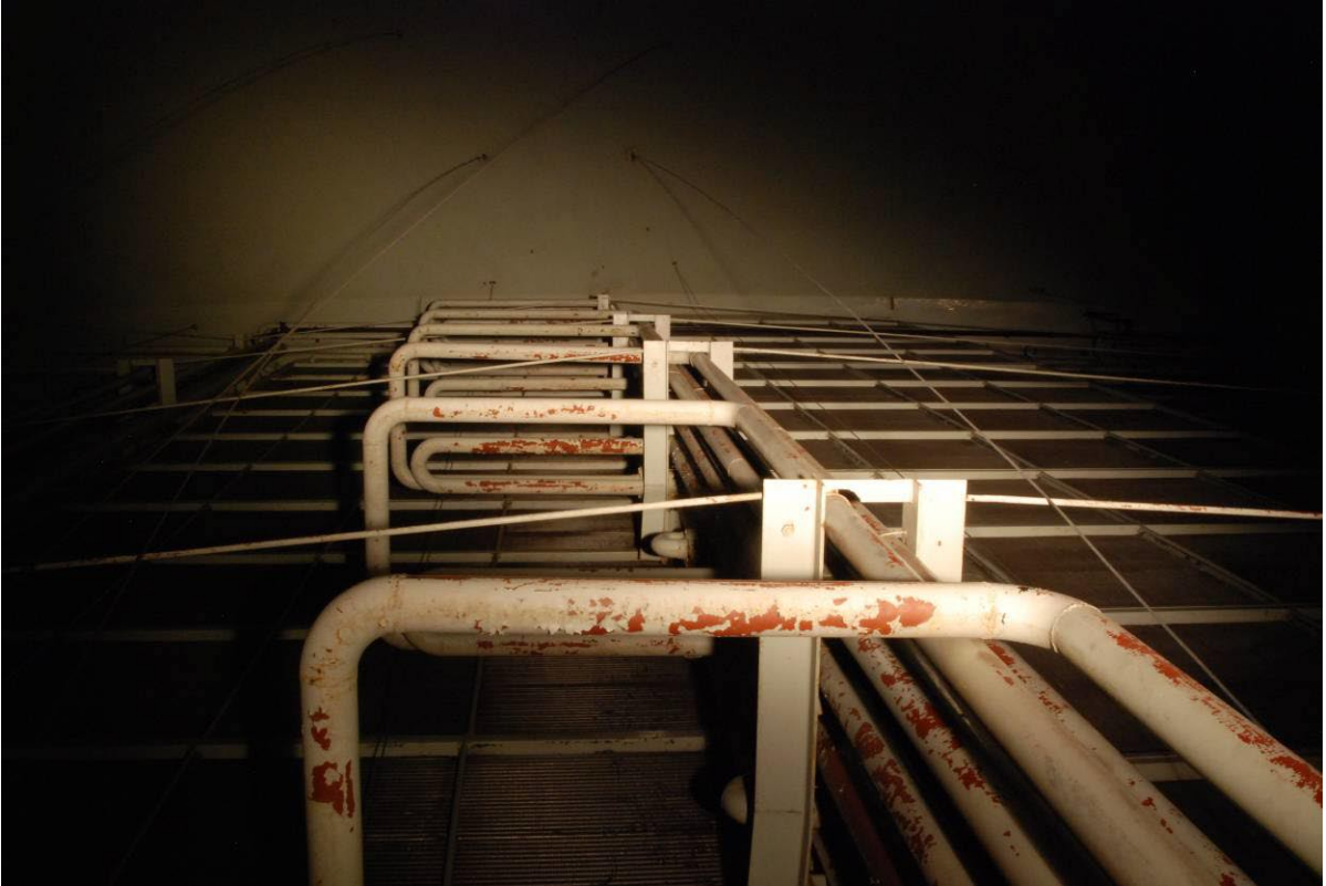
Figure 4: Looking Upwards at the Supply and Return Piping
